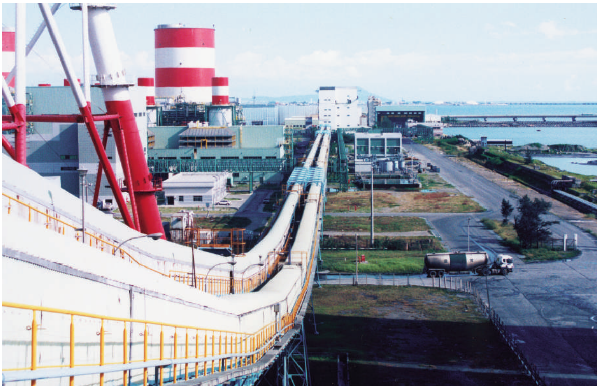
電廠輸送線 Conveyor Line at Power Station
